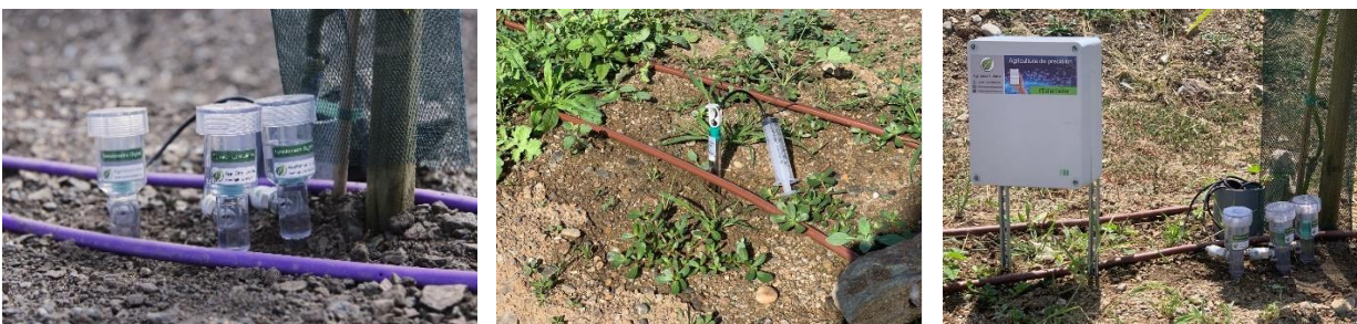
Figure 27. Tensiometers, lysimeters and iTelemeter components installed.
